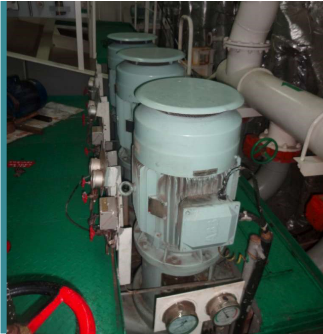
Machinery and systems shut down and preserved for cold lay-up
