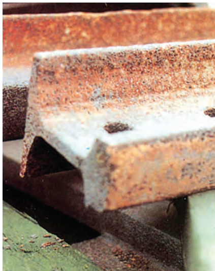
Fig. 12. Rails. Surface-condition clause: rust with pitting
