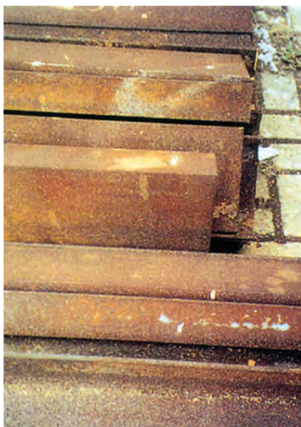
Fig. 9. Channels. Surface-condition clause: rusty
