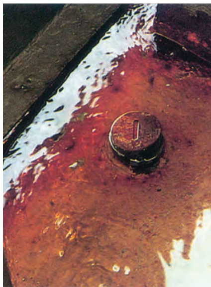
Fig. 27. Bilge sounding pipe surrounded by water. The pipe and its screw cap must be in good condition and the cap properly secured to ensure no water gets into the cargo hold below
