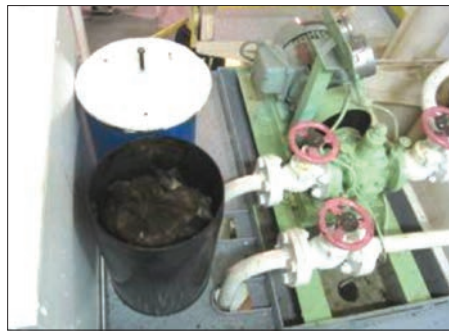
Rag bin with missing lid – a potential fire risk.
