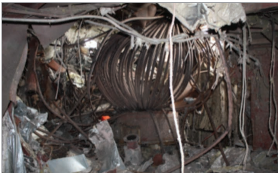
The aftermath of a boiler explosion.
