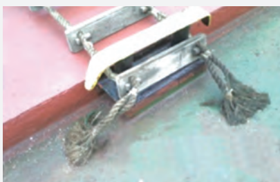
Photographs showing pilot ladders with no proper securing arrangements.
