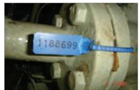
Figure: Sealed flanges
