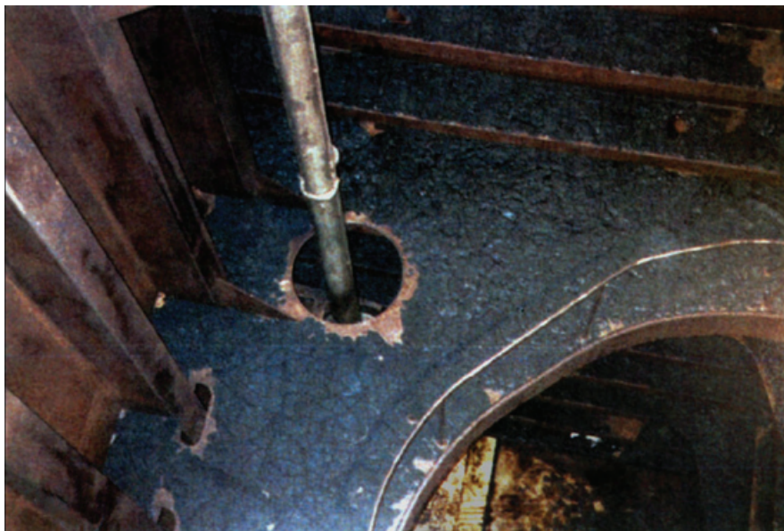
Fig. 5. Serious ROB problems caused by on-board blending of incompatible fuel oils. The remaining residue comprises precipitated asphaltenes which could not be removed by conventional water washing
