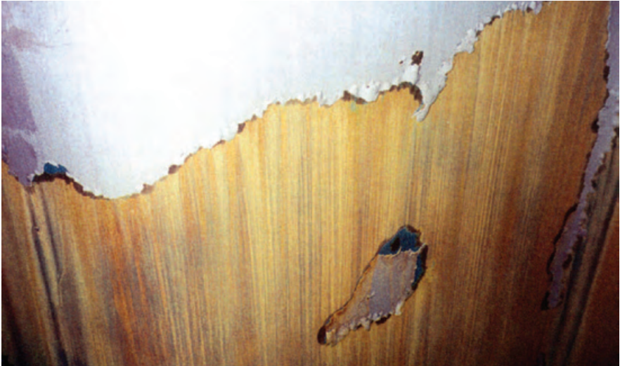
Fig. 14. New coating completely destroyed by an incompatible, aggressive cargo. The coating resistance was not referred to in this instance
