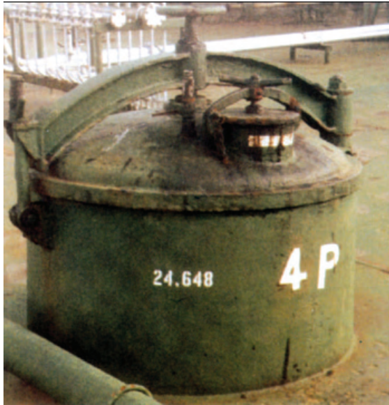
Fig. 4. The reference height of the tank has been clearly marked on this hatch coaming to assist the surveyor during cargo gauging. However, the retro-fitted vapour control valve (centre) is higher than the ullage port (right) to which the tank reference height relates. Ullage readings taken via the valve must thus be corrected before being entered in the calibration tables
