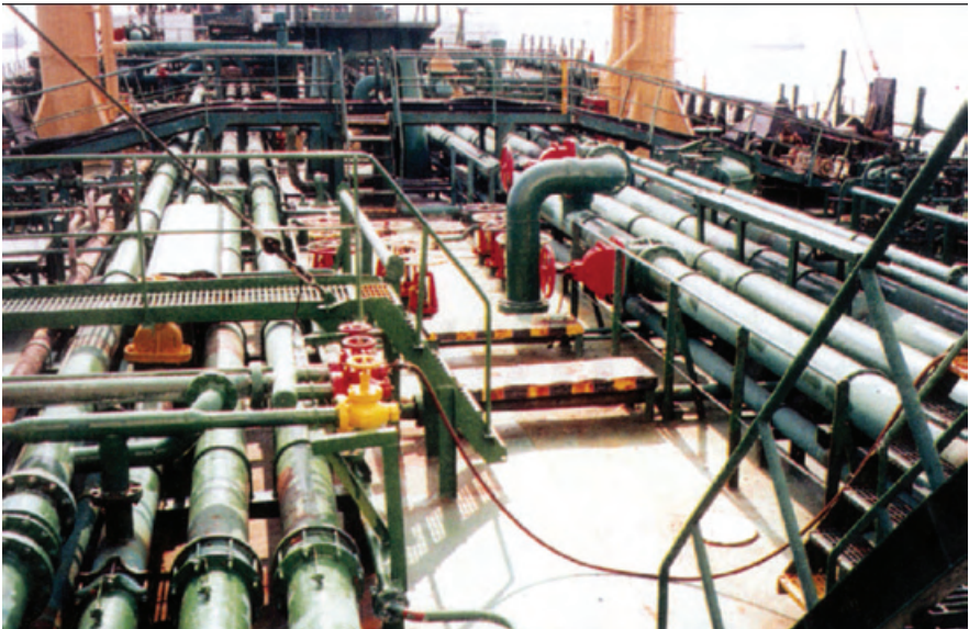
Fig. 15. The ship must ensure that all its cargo pumps, lines and fittings are free of potential contaminants
