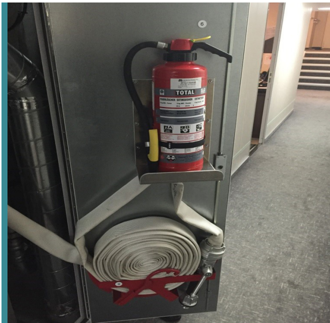
Fig 15: Planned maintenance should include both fixed and portable equipment
