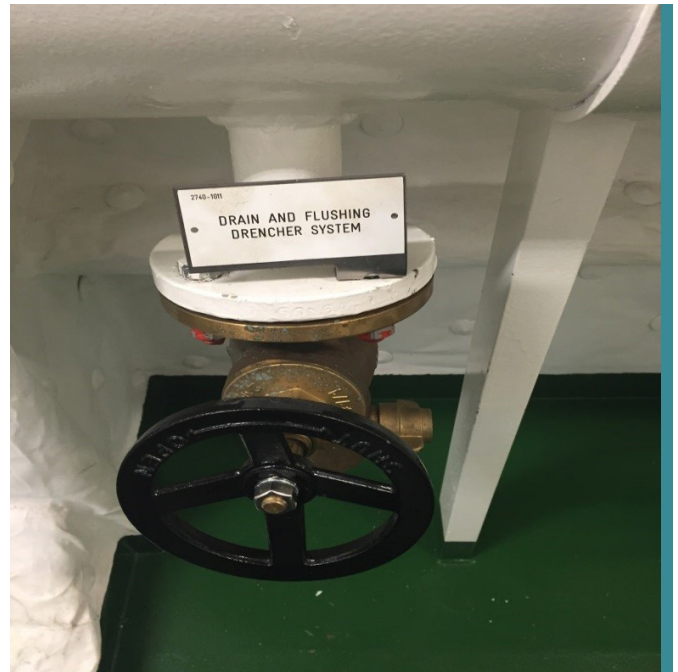
Fig 7: Drenching system flushing valve
