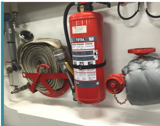
Fig 13: Portable fire-fighting equipment
