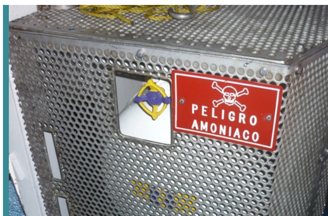
A well protected ammonia plant
