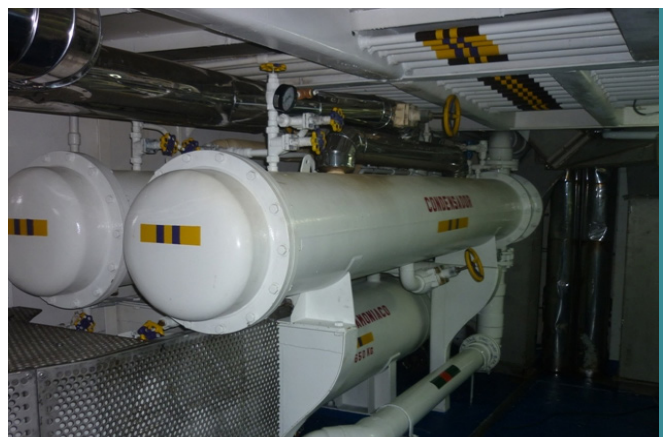
Ammonia receivers with colour coded pipework and protective grating around exposed parts
