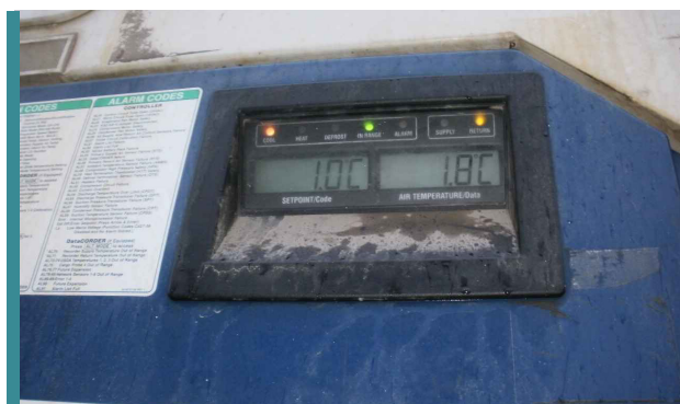
Figure 6: Monitoring of Reefer Temperatures
