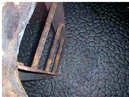
Fig. 14. Tank lid removed to reveal evidence of aerated 'cappuccino' bunkers
