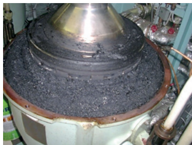
Fig 5. Unstable and incompatible fuel oils can lead to build-up of sludge (VPS)
