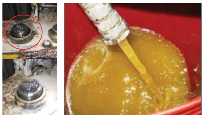
Example of contaminated oil and metal filings on the magnetic drain plug
