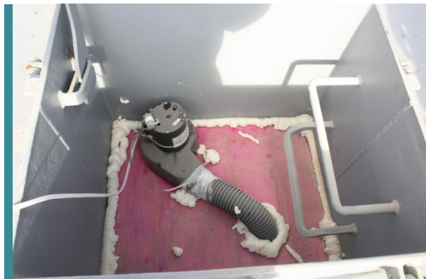
Recirculation fan positioned in hold access trunking
