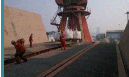
Steel meshed screen arrangement on hatch opening
