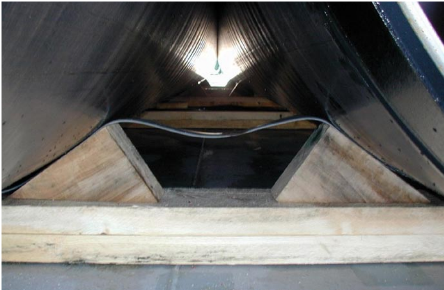
Fig. 4. Timber wedges nailed to base timbers are required along both sides of every pipe to prevent rolling
