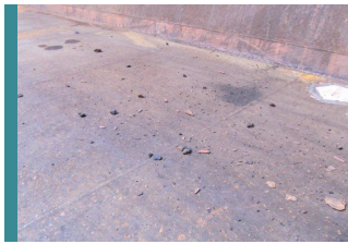
Not grain clean - loose rust and debris on tank top
