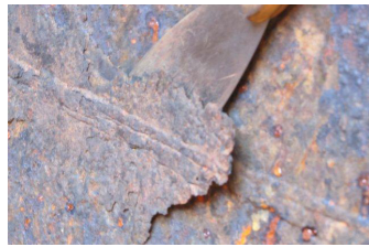
Not grain clean - loose rust found by survey
