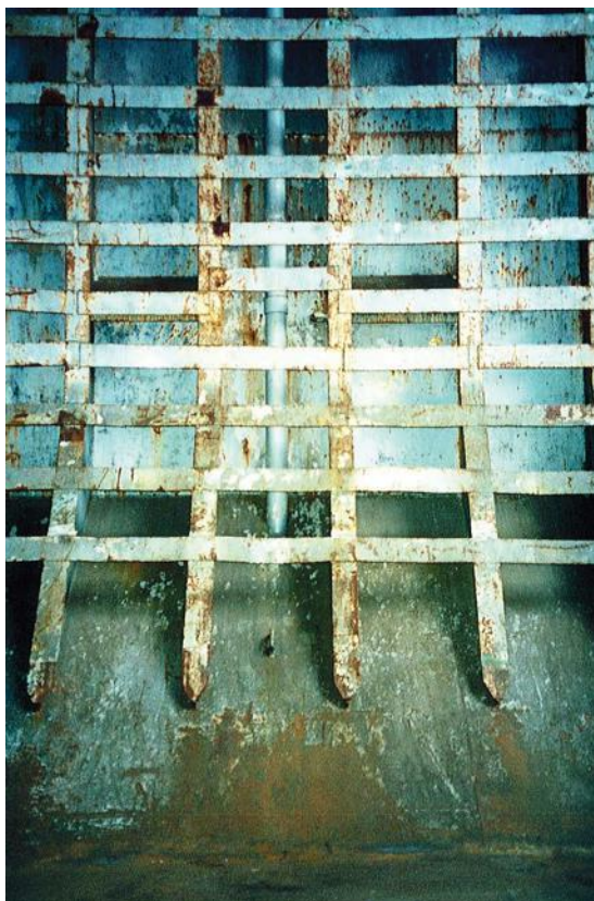
Fig. 18. Spar-ceiling can be permanently fitted in holds of ships that regularly carry bagged cargoes, helping to prevent cargo touching the sides of the hold
