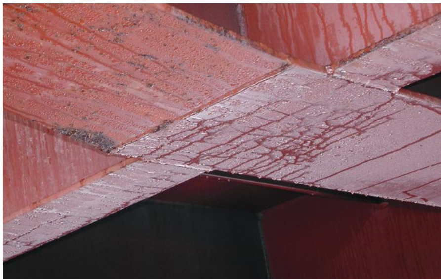
Fig. 1. Ventilation can prevent condensation or 'sweat' forming on hold steelwork and dripping onto cargo
