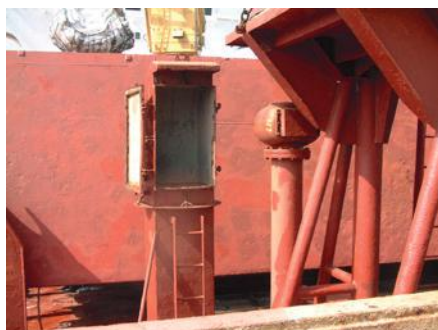
Fig. 23. Ventilators with vertical openings closed by a hinged door are a risk to cargoes, particularly if left open in heavy rain
