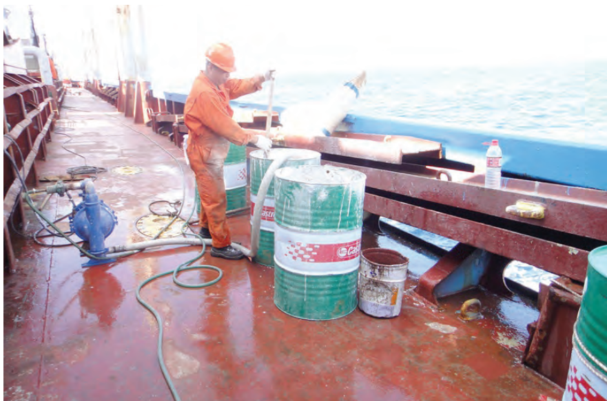
Fig. 11. Mixing lime and water in drums on deck for lime washing of the hold below
