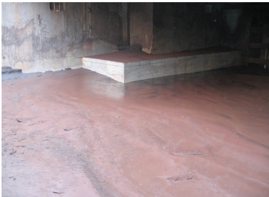
Fig. 24. The same stowage of chrome concentrate in Fig. 23 after it liquefied
