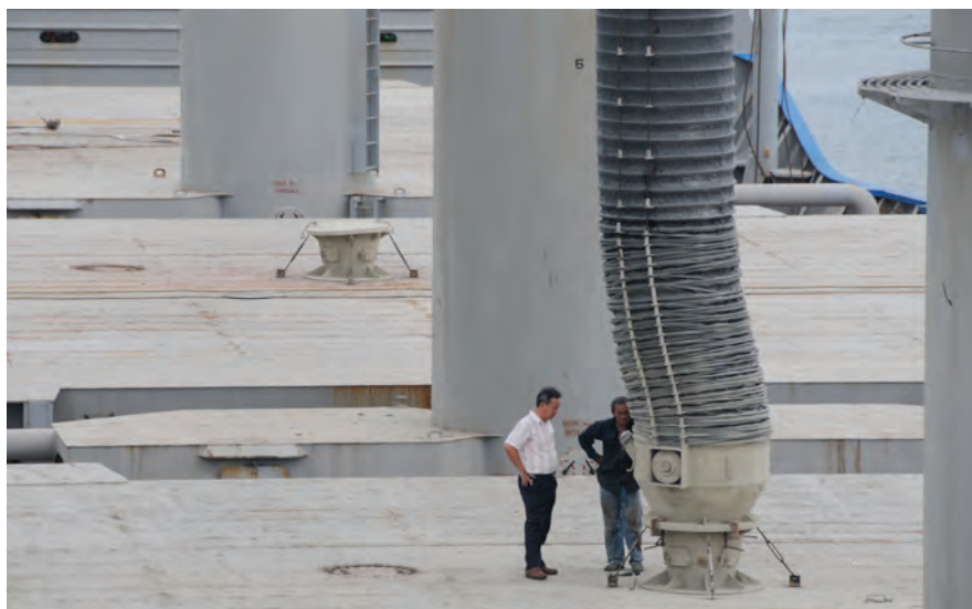
Fig. 30. Loading cement using pneumatic equipment via a cement port fitted in the hatch panel
