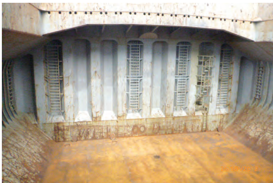
Fig. 16. The steelwork of the hold has been poorly maintained and displays extensive areas of loose rust scale and loose paint, and also areas of hard adhering rust scale
