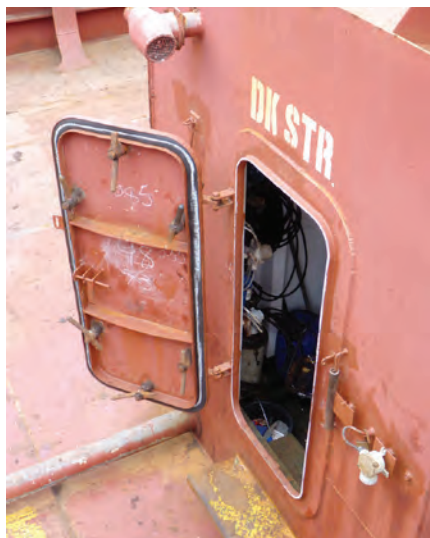
Fig. 7. A successful chalk testing of the weather door of a mast house
