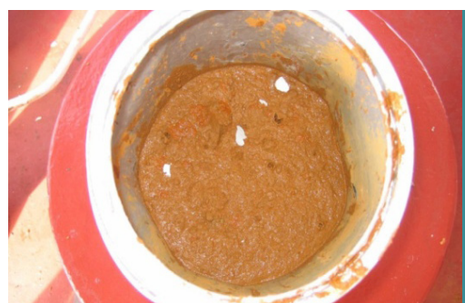
Figure 4: After - a failure on this occasion
