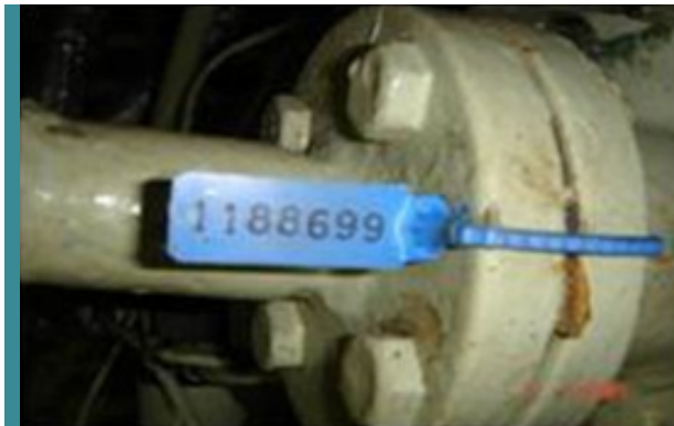
Security seals on flanges
